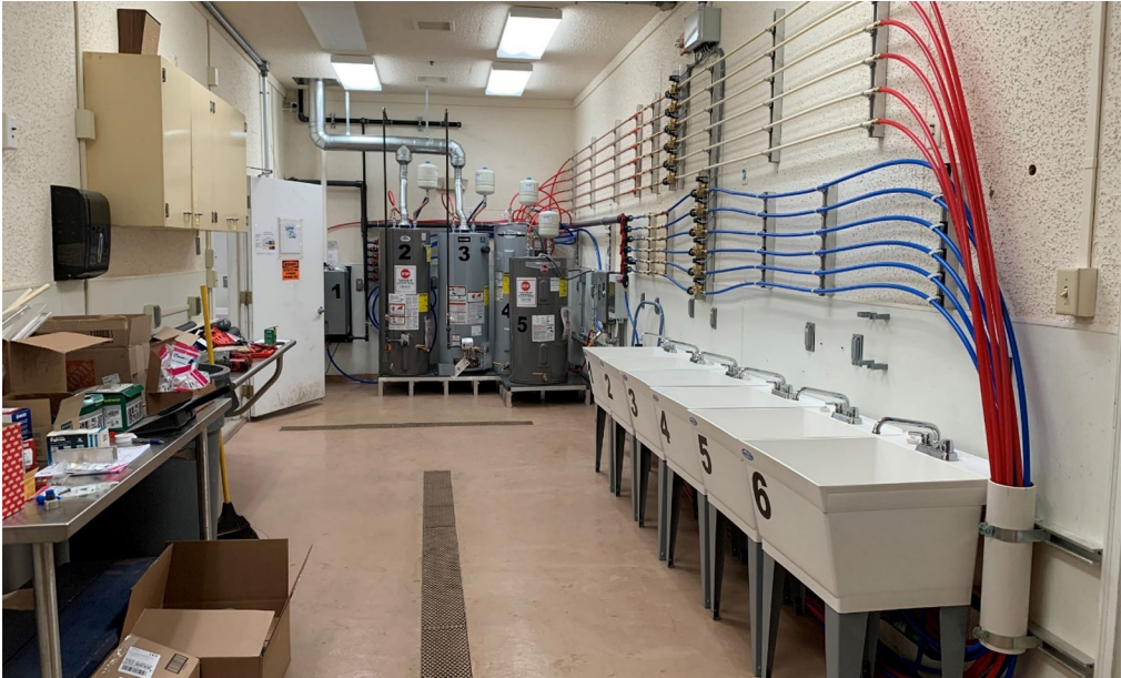
Full-Scale Premise Plumbing at the T&E Facility (1 of 2)
