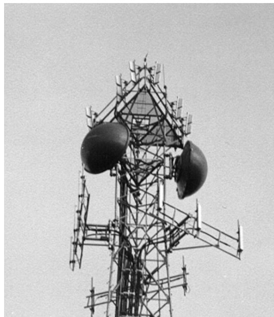
Figure 3b - Upper tower anemometer at a 187-ft (57 m) height above ground.
