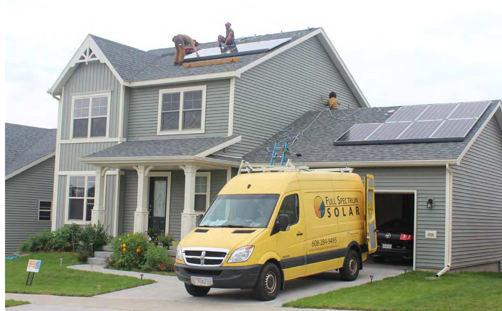
A residential participant has solar panels installed through the MadiSUN program with trade ally Full Spectrum Solar, a local small business in Madison.
