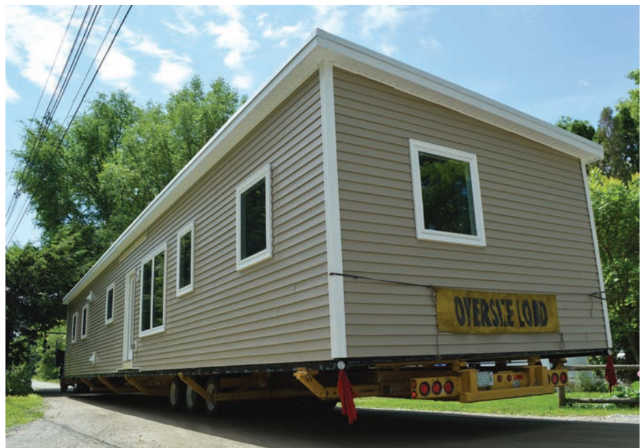
Modular homes are built inside a factory and transported using flatbed trailers and cranes for installation on a permanent foundation.
