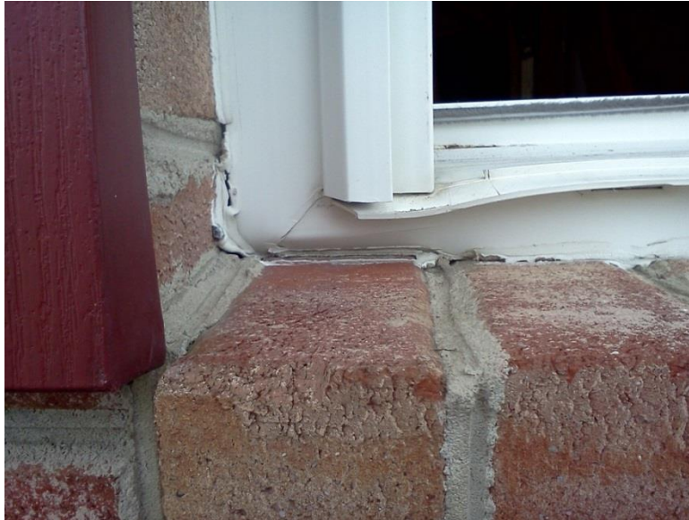
Figure 4–19: Deformed Window and Ruptured Caulking due to Shrinkage of Wood Framing
