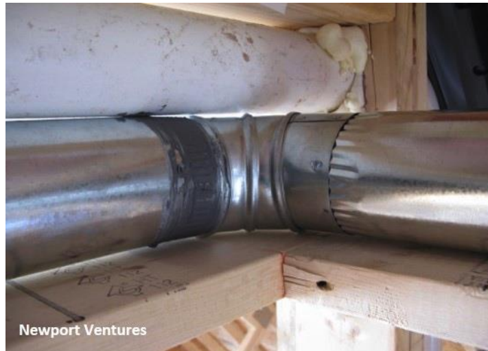
Figure 5–3: Example of Duct Joint Which Should be Air-Sealed
