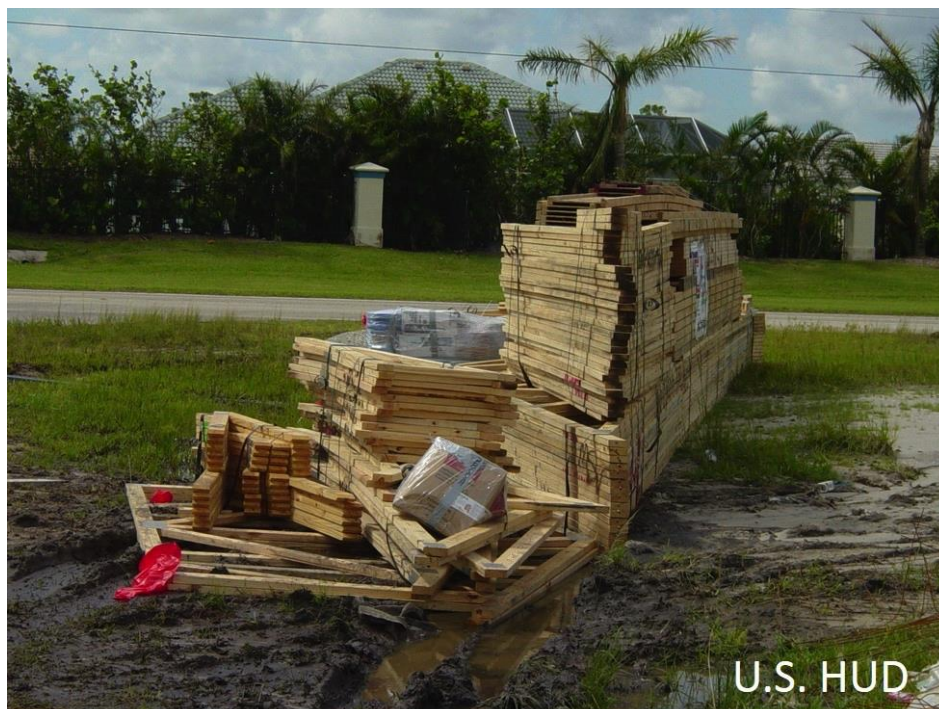
Figure 4–21: Example of Unacceptable Construction Material Storage
