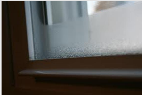
Window condensation is often a sign of elevated indoor RH levels.
