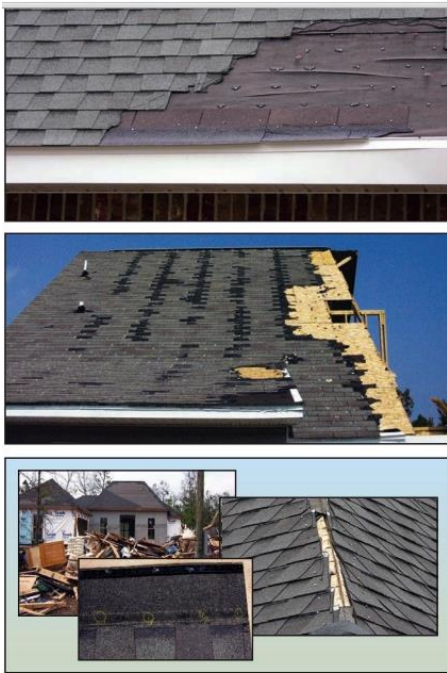
Figure 9-4: Examples of Roof Covering Loss
