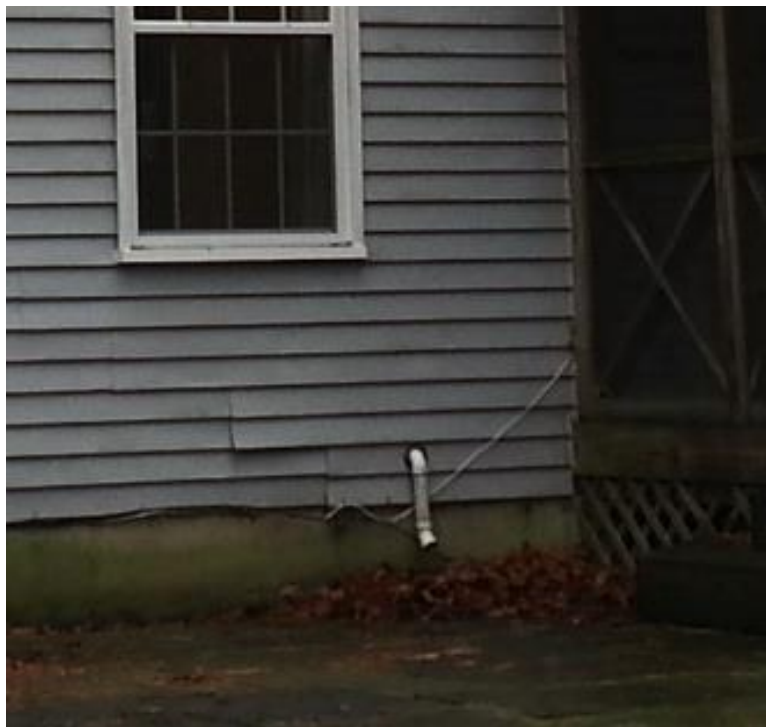
Figure 9–7: Sump Pump Discharge Right Next to Foundation
