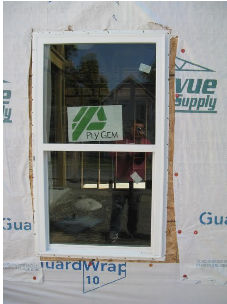
Figure 2–2: Non-existent Flashing Around Window, Practically Inviting Water Intrusion
