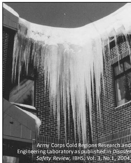
Figure 4–6: Example of a Severe Eave Ice Dam
