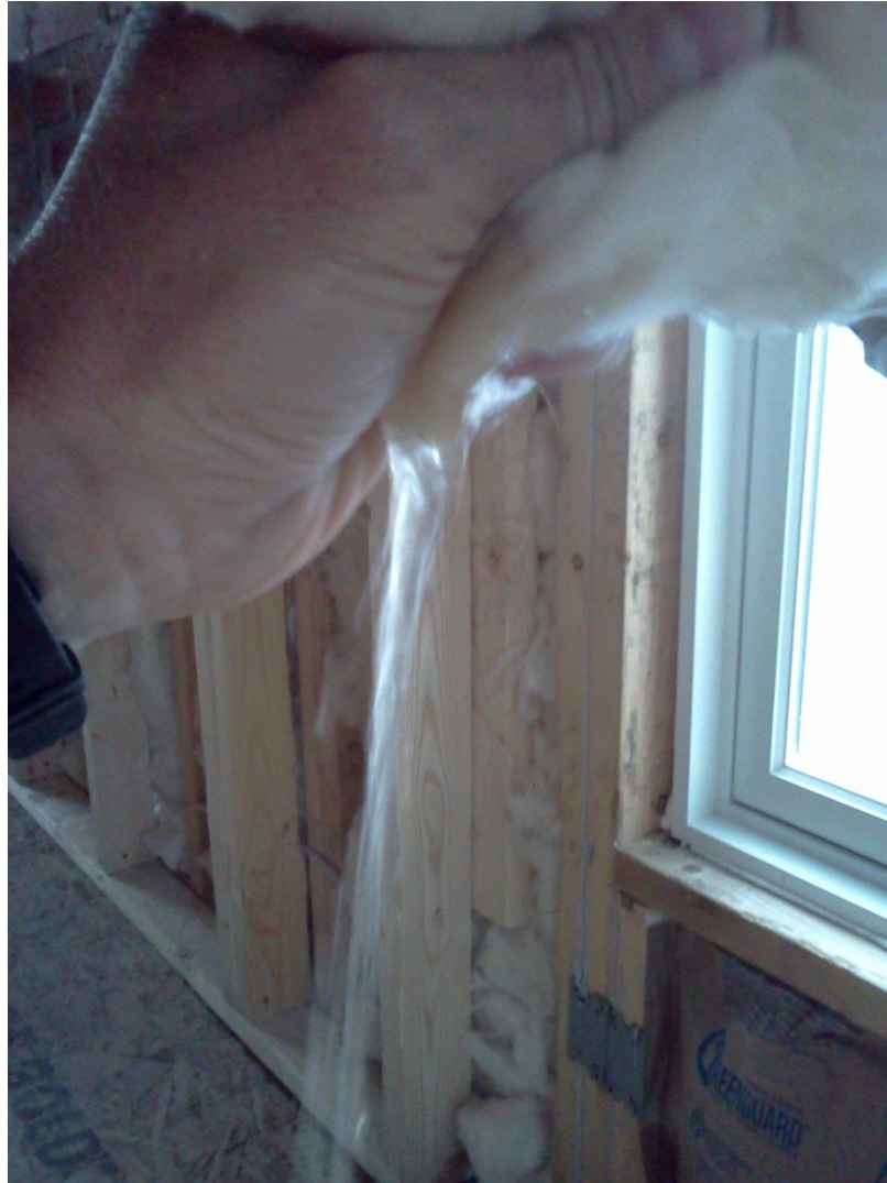
Figure 4–20: Water Streaming From Cavity Insulation as it is “Wrung Out”
