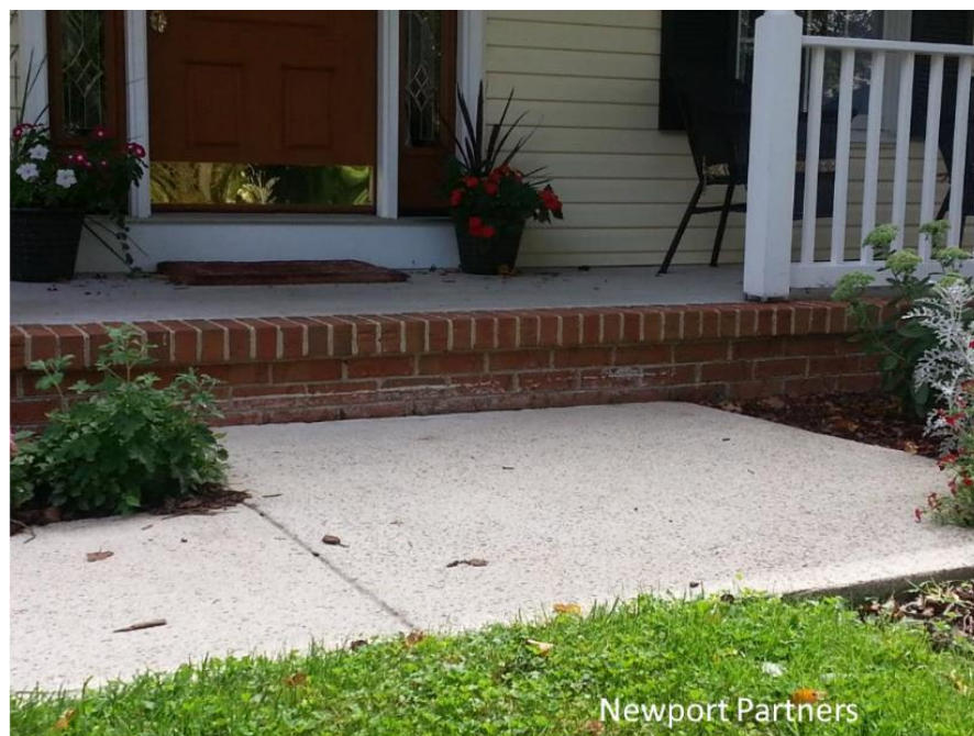
Front walkway which has settled due to insufficient compaction. Note the original concrete line against bricks, 3" higher than the current walkway elevation.
