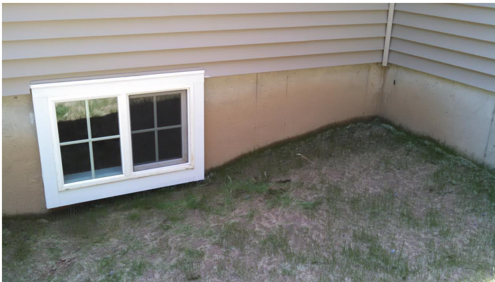
Figure 2–1: Soil Grade Slopes Towards the Foundation, Causing Water to Pool
