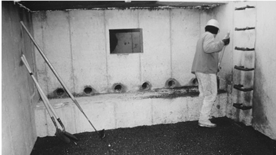
VIEW OF THE INSIDE OF A SAND FILTER SIMILAR TO THE ONE INSTALLED AT DUKE STREET SQUARE
