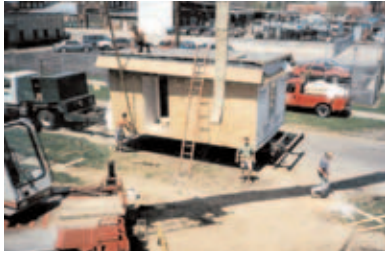
Modular housing arrives on the site as nearly finished modules (courtesy, MHI).
