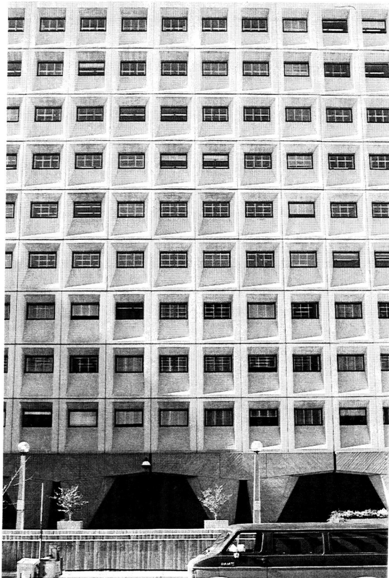
Illustration No. 4-10 Subject: Housing and Urban Development Building, Seventh Street (East) Elevation Date: November 1994 Description: View looking west with garage entrance walls in foreground (see Illus. No. 3-46 for original view). Note soiling on window units above glass and contrast of white replacement tape used on window Venetian blinds. Original blinds were 2" wide baked on gray flexible steel Venetian blinds with 1-1/2" wide gray tapes and gray nylon cords. Note also non-original spotlight mounted on center of beam between pilotis, new glass globes and signs on original concrete standards, and concrete landscaping planting boxes. Photographer: Reed A. Black, AIA Source: Oehrlein & Associates Architects
