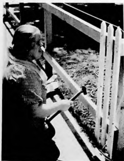
To keep construction and renovation costs down, tenants do much of the work themselves. Yet cost-consciousness does not necessarily mean spartan surroundings. A new picket fence will grace the front yard of this townhouse, one of 16 renovated by Community Corporation on Kansas Street.
