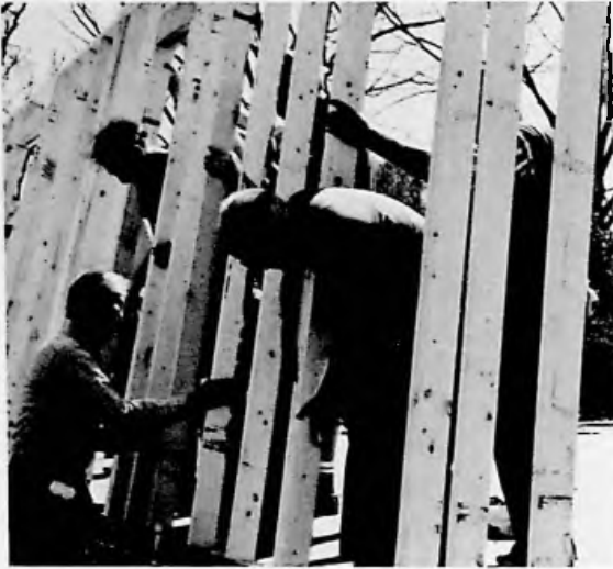
In Americus, Georgia, site of Habitat for Humanity headquarters, volunteers—including former President Jimmy Carter—help erect a new home for one of the area's very-low-income families. Americus is also the site of Koinonia Farm, an interracial community where the idea for Habitat for Humanity was first conceived.
