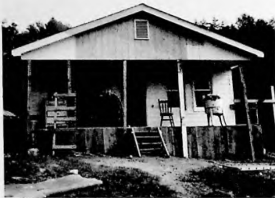
Repair of the Otis Smith house approaches completion. Kentucky Mountain replaced the insulation, siding, interior walls, windows, and floors.
