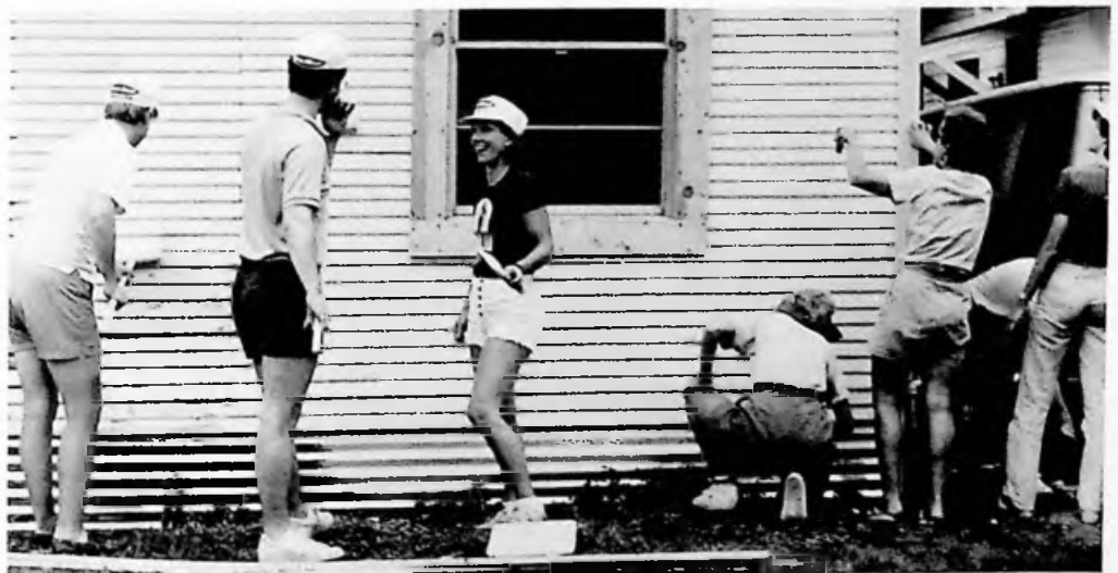
Volunteers from Highland Park United Methodist Church work on a home Common Ground renovated in Dallas' Fair Park area. Such volunteer efforts, together with donated materials, help Common Ground cut rehabilitation costs.
