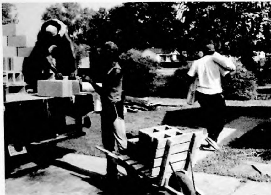
Most rehabilitations involve substantial structural repairs, including shoring up or completely rebuilding foundations.
