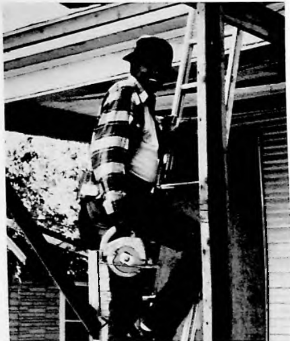
Roofing contractor Clay Williams works on one of the houses Common Ground is rehabilitating in Dallas. All Common Ground renovations are done by minority contractors.
