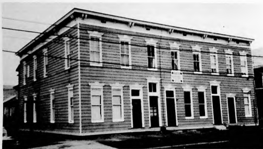
This old, dignified building at 62-68 North Champlain Street was badly in need of repair when this photo was taken. The Land Trust saw its potential as a housing cooperative and so acquired and renovated the building. Now six resident families jointly own the building and lease the land from the Land Trust.
