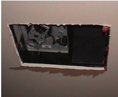
Figure 43 Paper tear in ceiling panel
