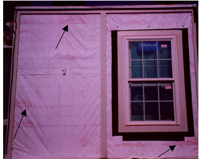
Figure 11 Conventional Fiber Cement Specimen - Clear Wall
