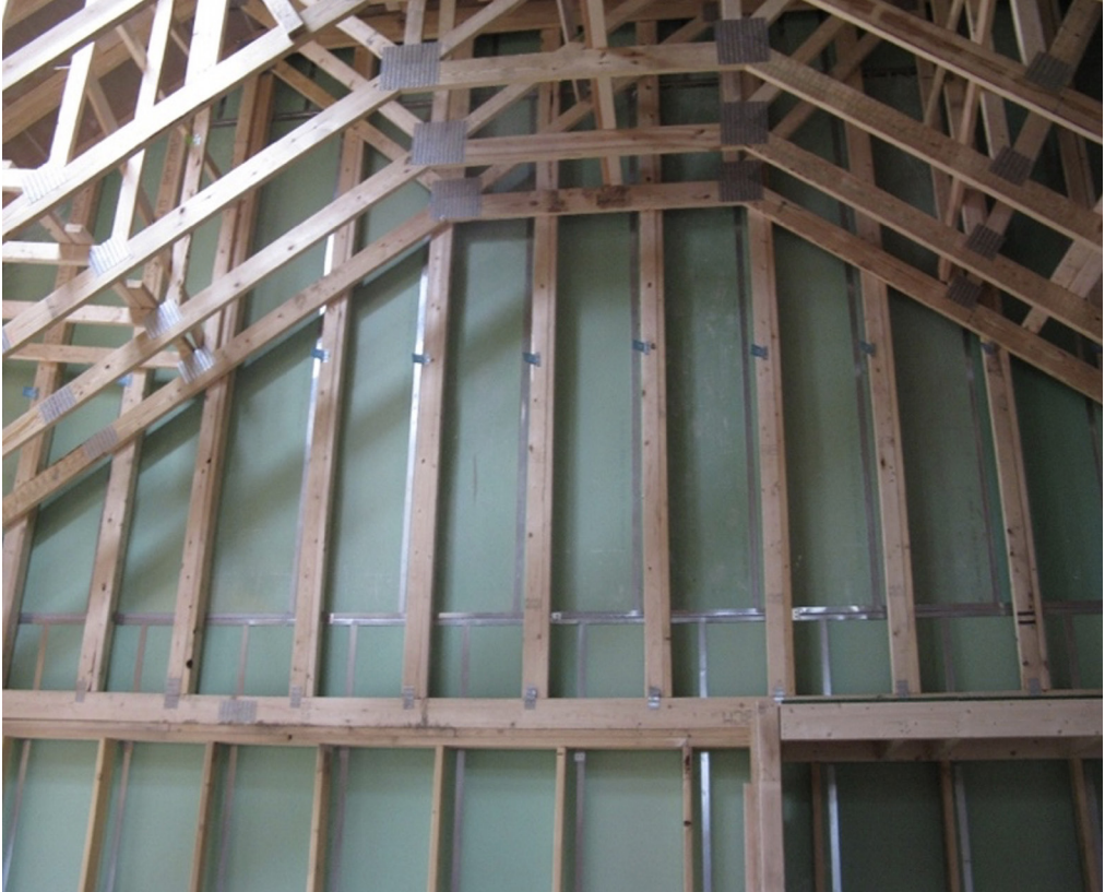
Example of a 2-hour fire-rated gypsum shaftliner assembly. Photo credit: Newport Partners.
