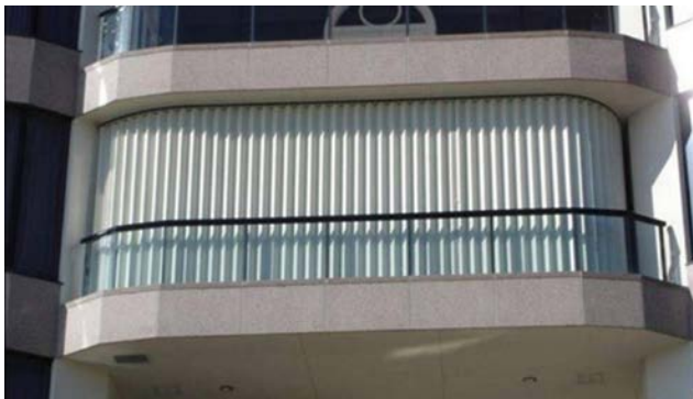
Accordion or other high-quality shutters protect glass from intense winds and flying objects. Photo courtesy SecurityRollingShutters.com .
