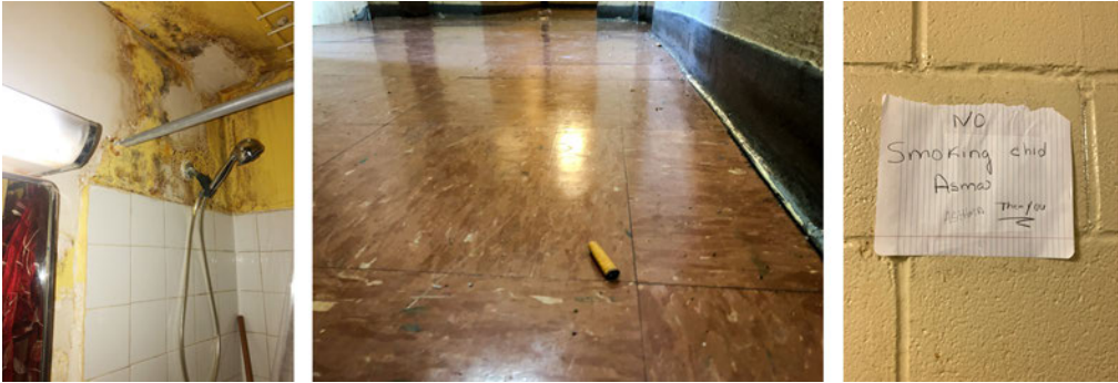
Notes: Images, from left to right: (left) bathroom in disrepair with a long-term water leak and black mold; (middle) cigarette filter and other debris in a hallway serving as evidence of smoking in common areas of the building; and (right) sign in a hallway that read "No Smoking chid Asma Than you" [sic]. Source: HaRBOR study team
