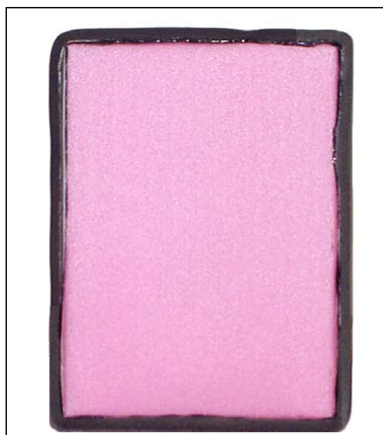
Figure 4 Attic Hatch with Perimeter Cushion
