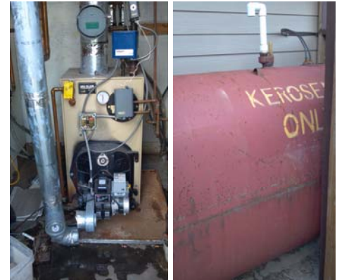
Figure 3 & 4: Boiler & Kerosene Oil tank for a Phase 1 building.
