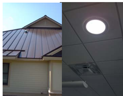
Figure 10: Solar tube lighting for a Phase 2 building outside (left) and inside the unit (right).
