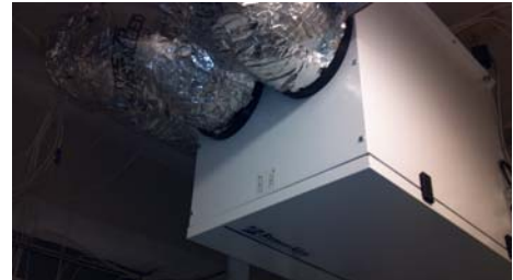
Figure 8: HRV system for the Phase 2 buildings.
