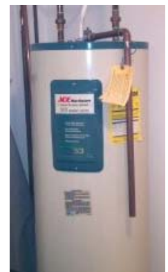
Figure 5: DHW tank for a Phase 1 building.
