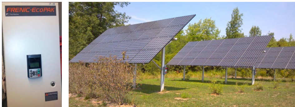
Figure 22: Inverter (left) and photovoltaic system for Phase 2 buildings (right)
