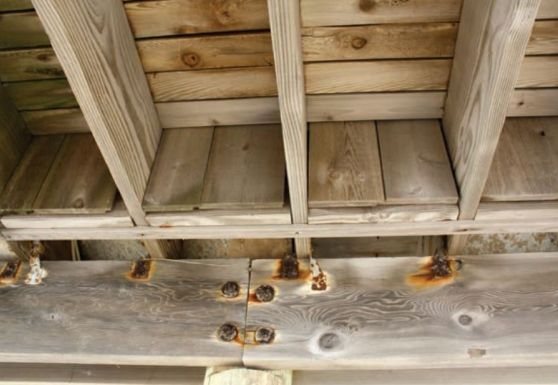
Corroded metal connectors and fasteners. Source: NFIP Technical Bulletin 8
