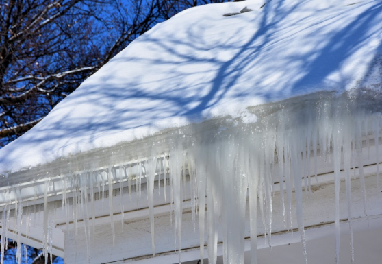
Meltwater can be trapped behind ice dam and seep under shingles.
