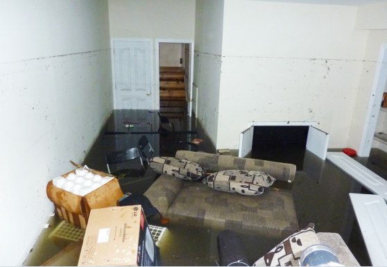
Damage to wall components due to bulk water and water infiltration.
