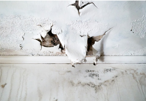
Damage caused by water intrusion due to roof failure.
