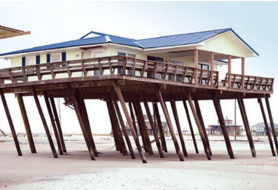
Damage from Hurricane Katrina in the Gulf Coast.
