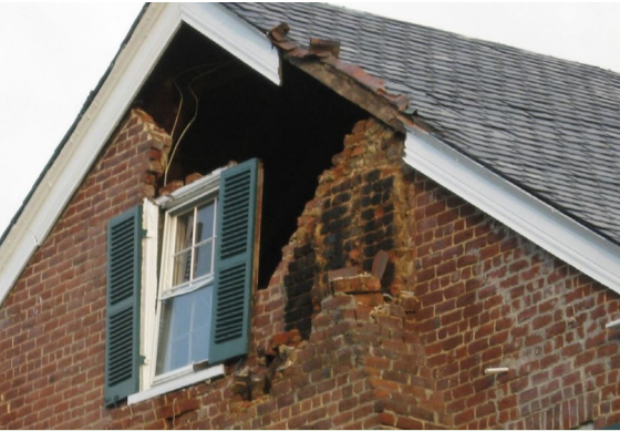
Failure of gable wall. Source: FEMA P-530
