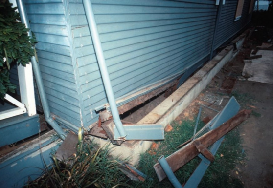
Watsonville, California, 1989 Loma Prieta earthquake. Source: FEMA P-749: Figure 17
