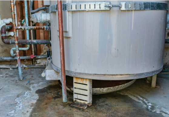
Leakage following a water heater pipe break.
