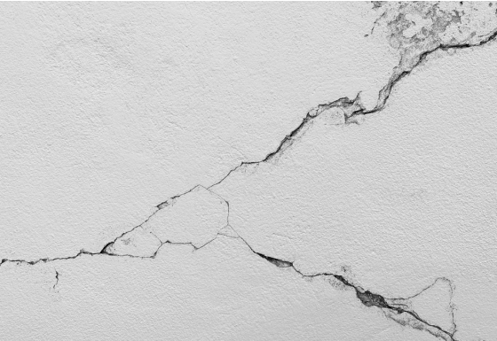
Failure and damage to masonry cladding.
