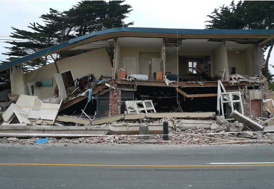
Failure due to lack of load path. Source: U.S. Geological Survey
