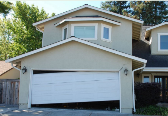
Garage door damage. Source: FEMA P-530
