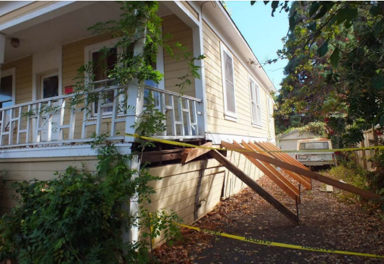
Damage to cripple wall. Source: FEMA P-1045 Photo Credit: Estructure
