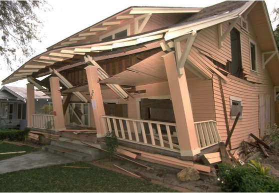
Failure of building wall and floor. Source: Mitigation Ideas (FEMA)
