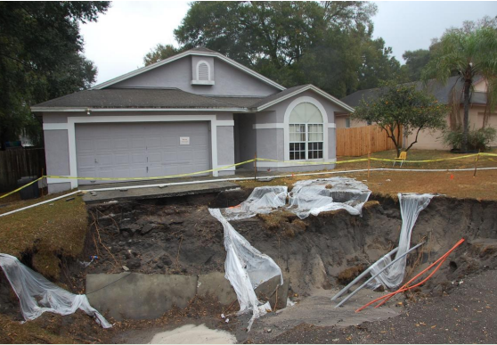
Sinkhole damage. Source: U.S. Geological Survey
