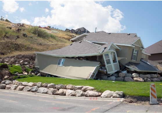
Two-story vaulted area failure.
