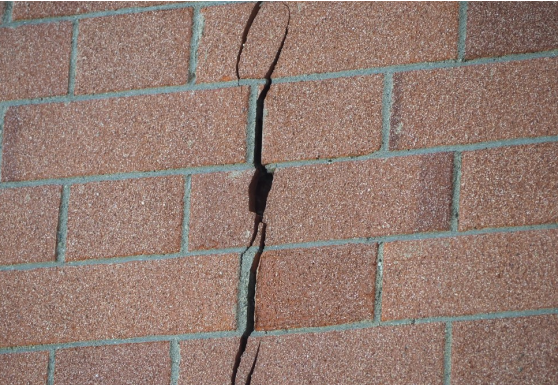
Brick veneer damage.
