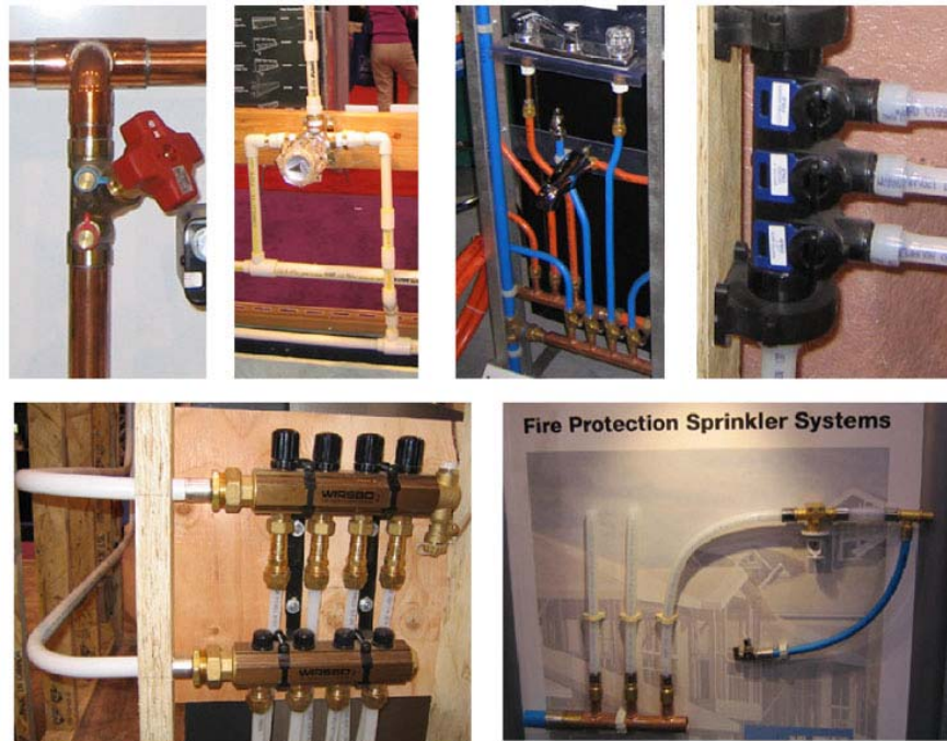
Clockwise from top left: traditional soldered copper pipe, glued CPVC, PEX and copper, PEX with plastic fittings, PEX with metal fittings, and PEX used for sprinkler systems. Photos from International Builders Show.
